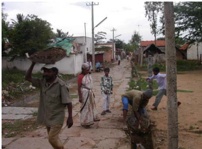
Channapatna, slum residents cleaning the drains.
